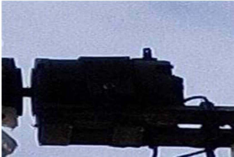
Gambar 4.5 Generator (Sumber :Penelitian 2020)
