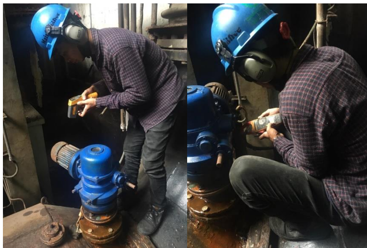
Gambar 4.7 Pengujian Motor Debris Filter
